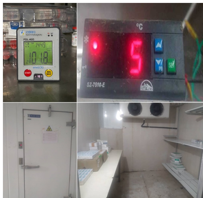
Figure 73. Cold room and data logger
